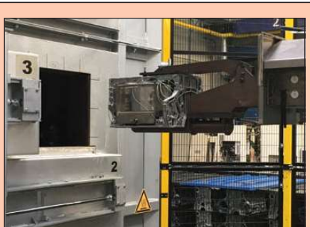
Fig.14: Robot loading of combined 'thru-process' system with engine block into BSN rotary T6 furnace. The thermal barrier is designed with a combination of thermal insulation technology capable of fitting in the engine block cavity. With a thermal protection capability of 550°C for several hours, the system has the ability to monitor the complete T6 process, including solution reheat, water quench and aging.
