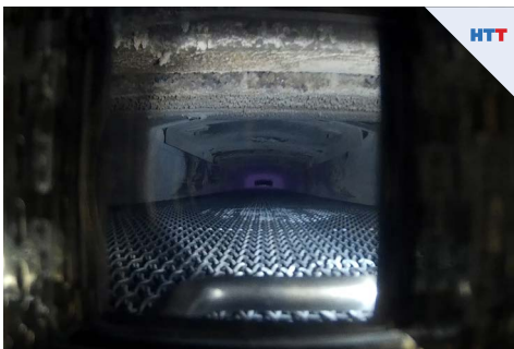
Figure 5.2. Video image in inner CAB furnace showing condition of inner furnace, mesh belt and product transfer
